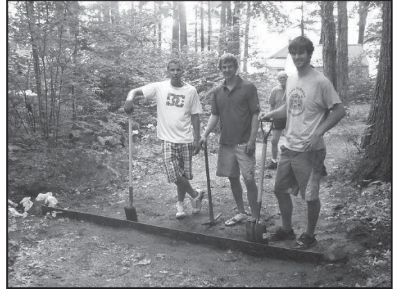
RWPA Lakes Rangers take a day off from inspecting boats to install a rubber diverter on a road. Rubber diverters help direct water into vegetated areas and away from the lake.
